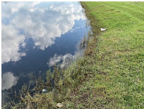
Minor shoreline erosion
