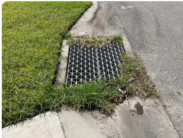
Debris accumulation near catch basin
