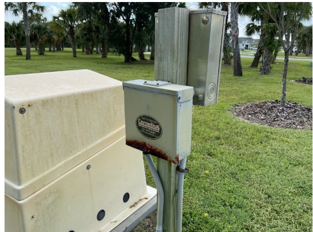
Rust at electrical panel
