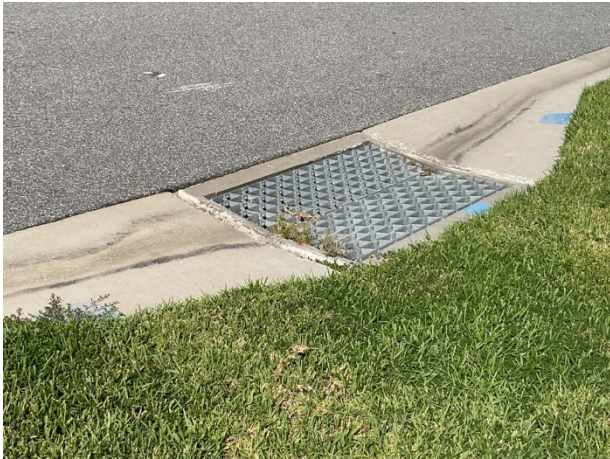
Catch basin collar damage
