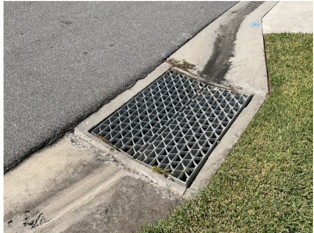
Catch basin collar damage
